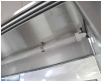
Top mounted fluorescent lighting
